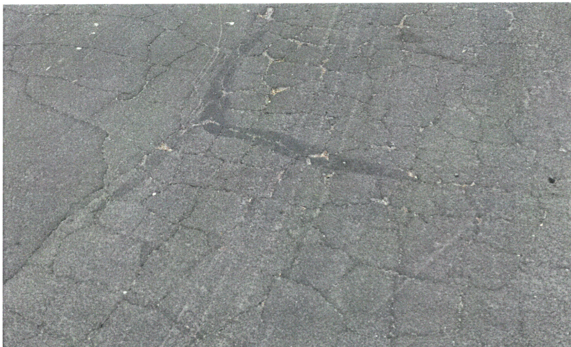
Figure 7 Example of Fatigue Cracking
