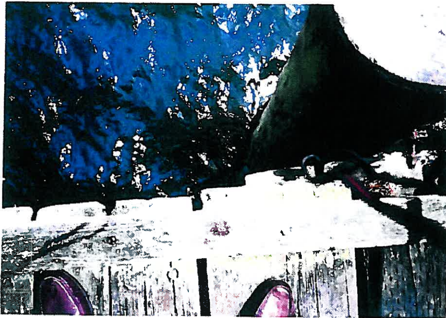
FENDER PILE BROKEN AT WATERLINE PHOTOGRAPH NO. 8
