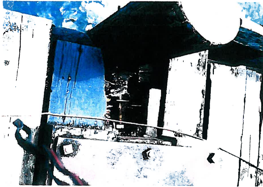
FENDER PILE CONENCTION DAMAGE AT DECK LEVEL PHOTOGRAPH NO. 7
