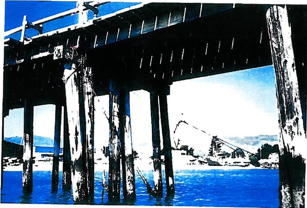
VIEW OF PIER FROM WATER AT GRIDLINE 20 SHOWING FRAMING PATTERN LINE (NOTE CABLES HOLDING PIER) PHOTOGRAPH NO. 3
