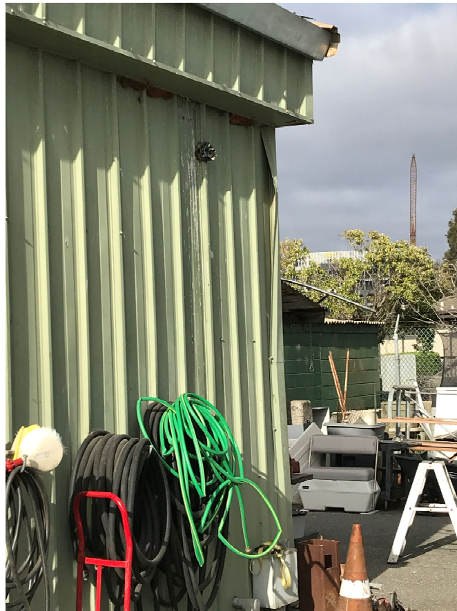
53 – View of warped northwest corner of Maintenance Building
