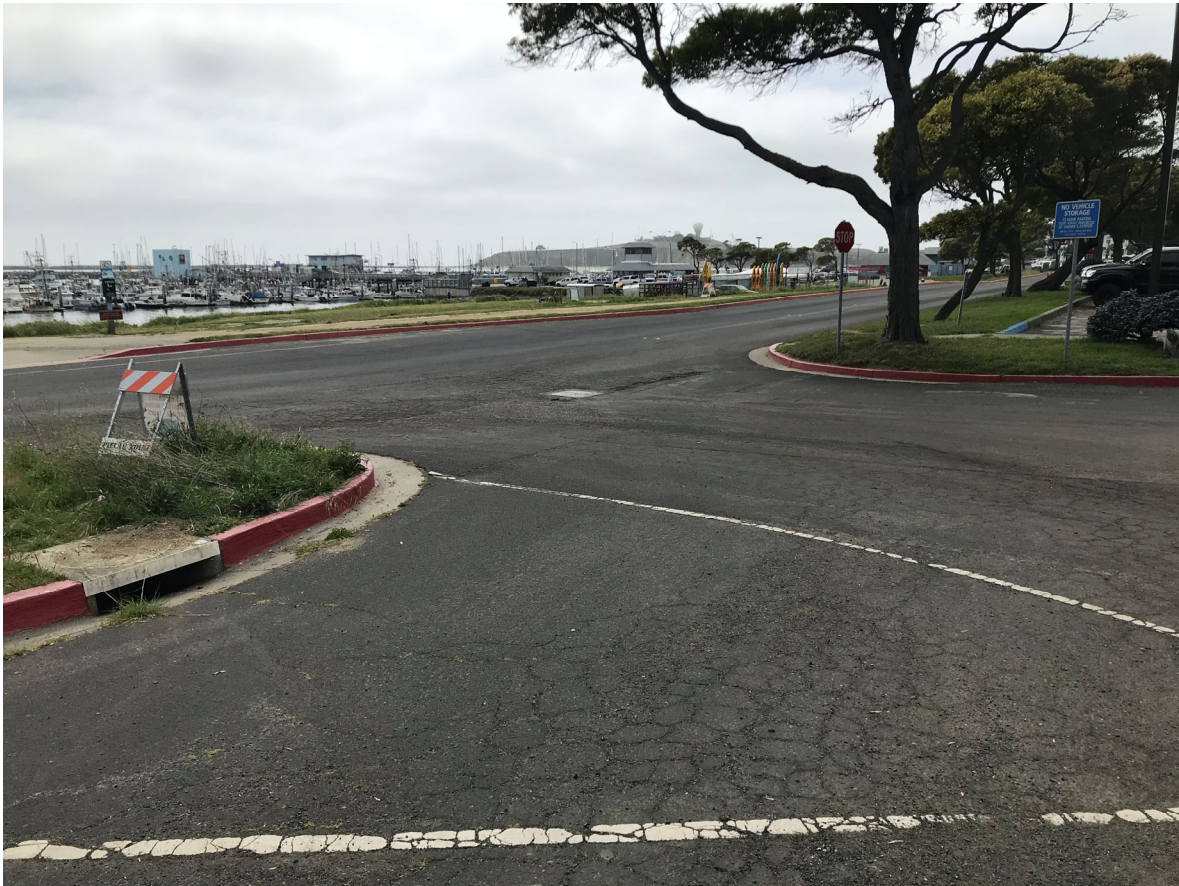
48 – View of worn and failing pavement to boat trailer parking area
