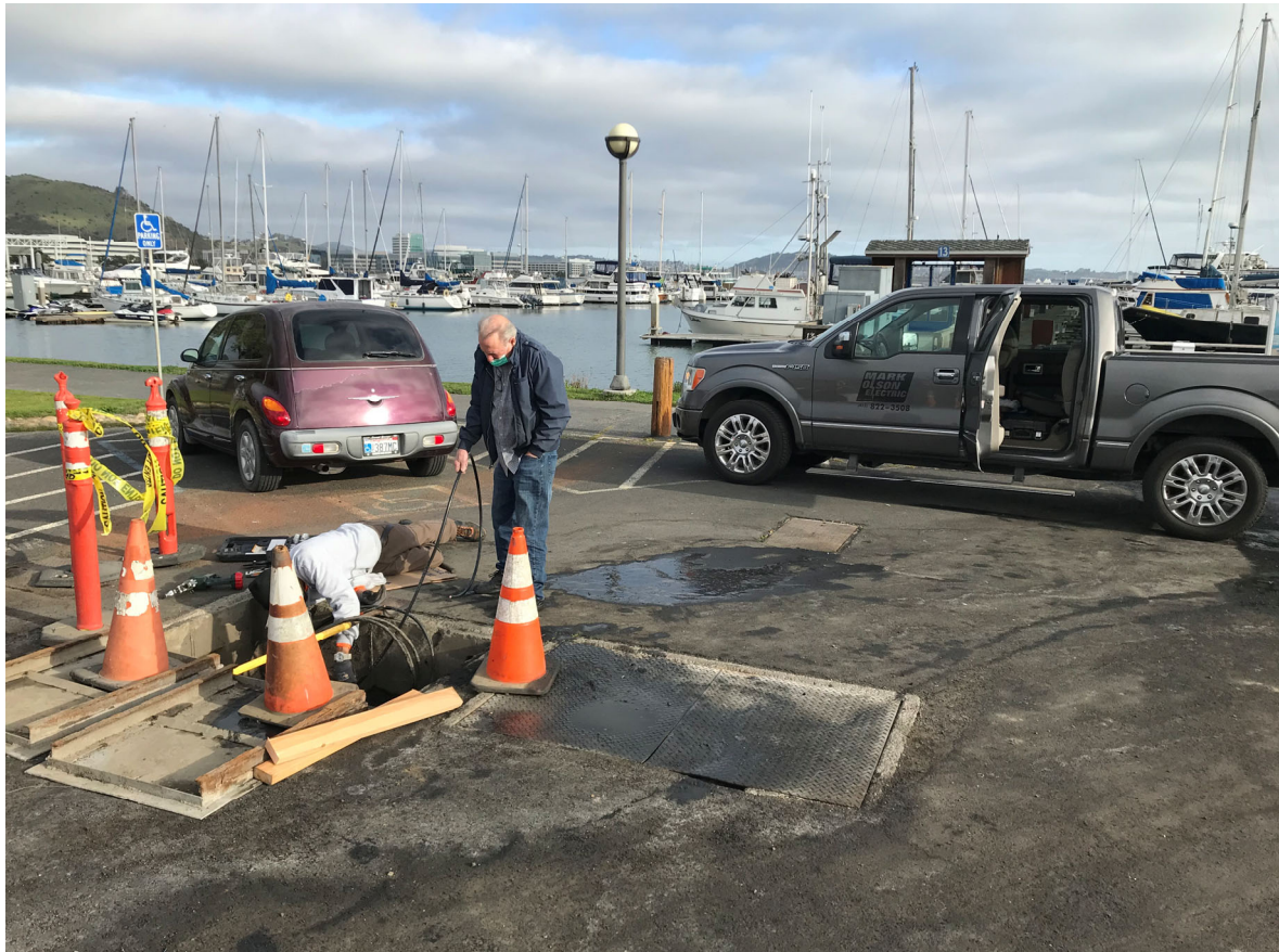
77 – View of electrical vault near Dock 13 being maintained
