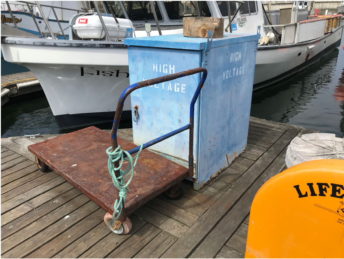
62 – View of Dock E electrical transformer
