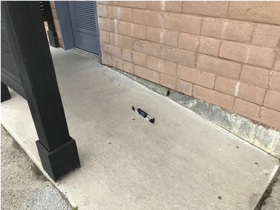
27 – View of West Restroom concrete ramp to shower room (does not meet ADA slope requirements)
