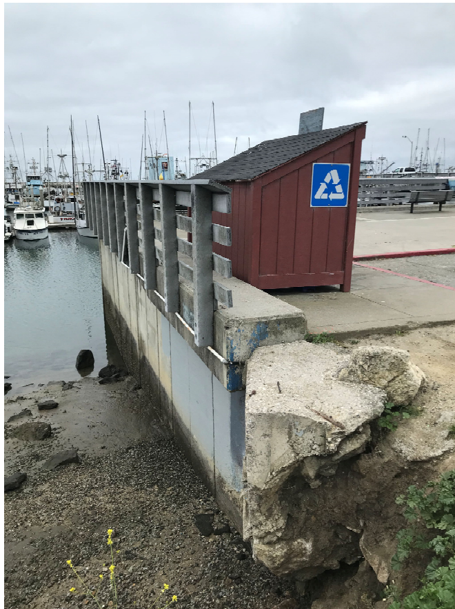
19 – View of promenade and east end of sheet pile wall (with exposed concrete block)
