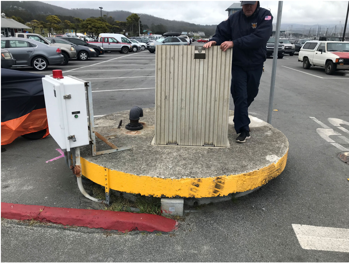
36 – View of sewer lift station in Parking Lot A
