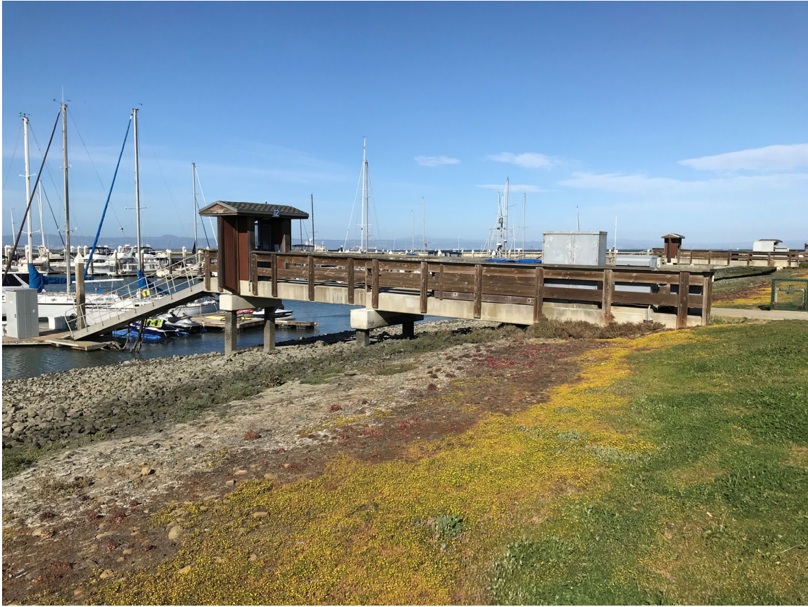
32 – View of Dock 12 gangway platform
