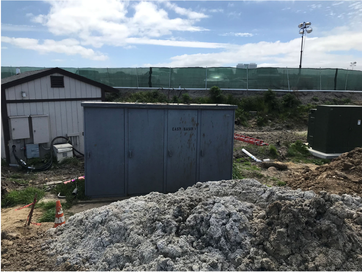
72 – View of Edison and Marina electrical distribution enclosures next to Vacuum Building
