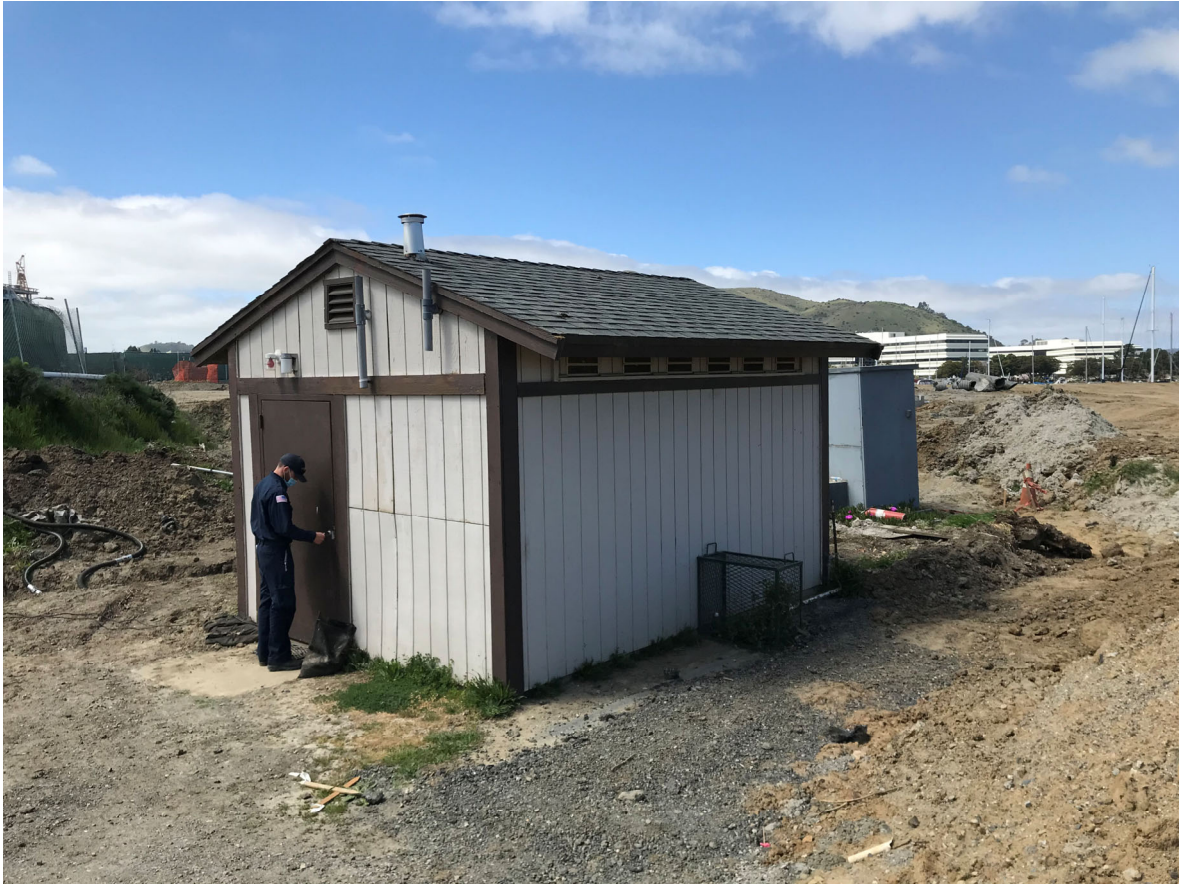
70 – View of Sewer Vacuum and Ejection Building (lift station) and surrounding new site grading
