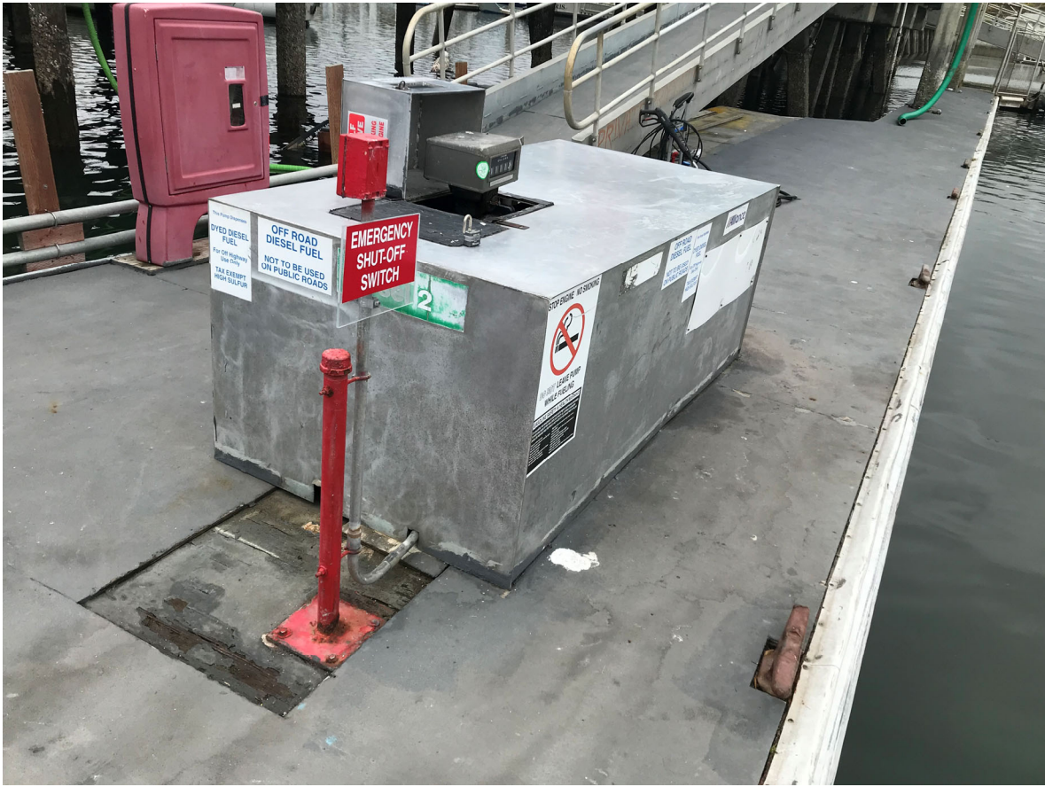
72 – View of Fuel Dock dispenser and emergency shut-off switch
