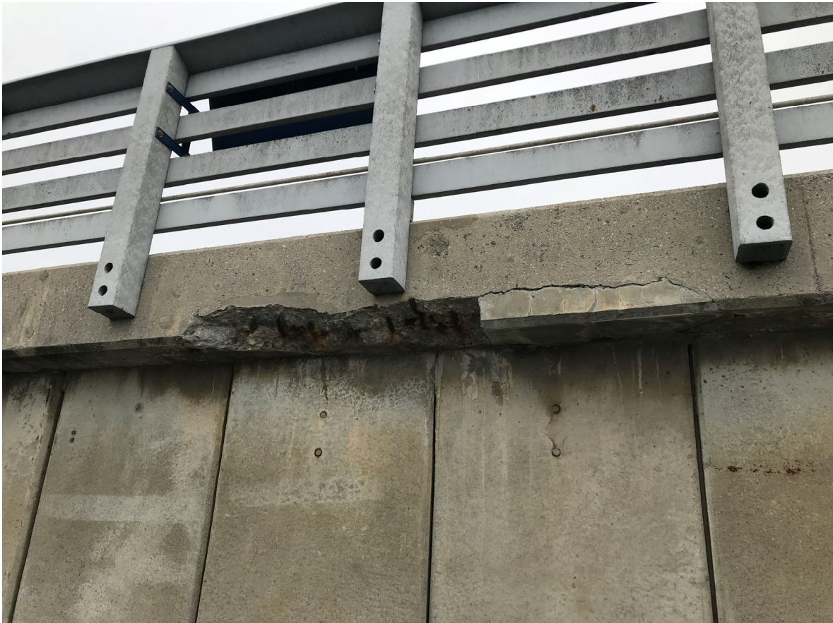
21 – View of distressed sheet pile wall concrete cap
