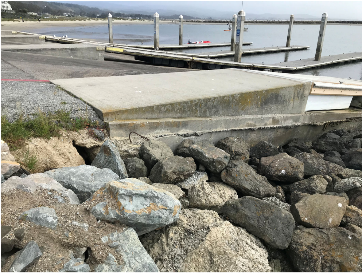
46 – View of boat ramp abutment undermining
