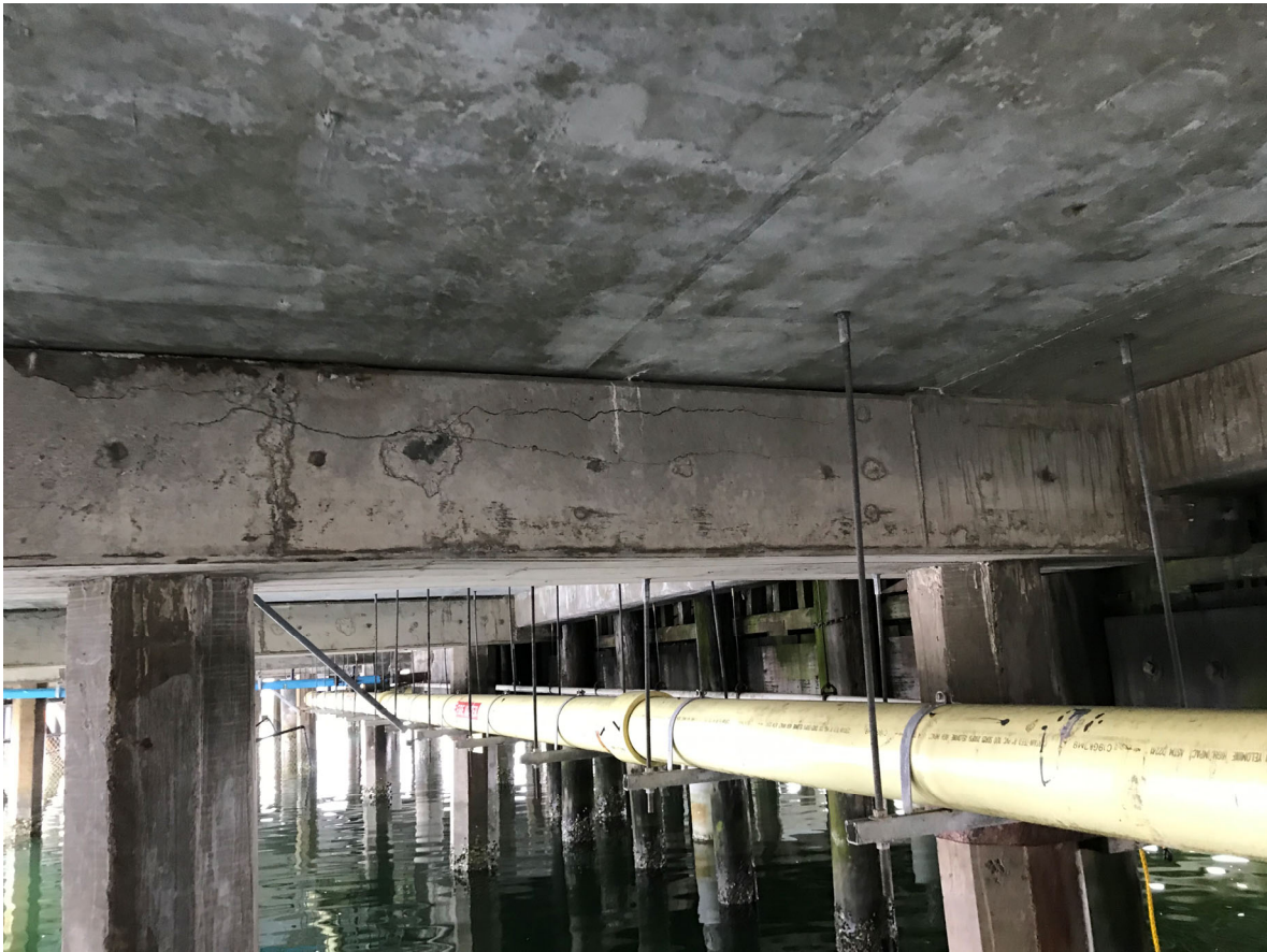
8 – View of overstress cracked beam and utilities under end of pier
