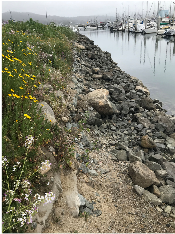
24 – View of failed rock slope protection
