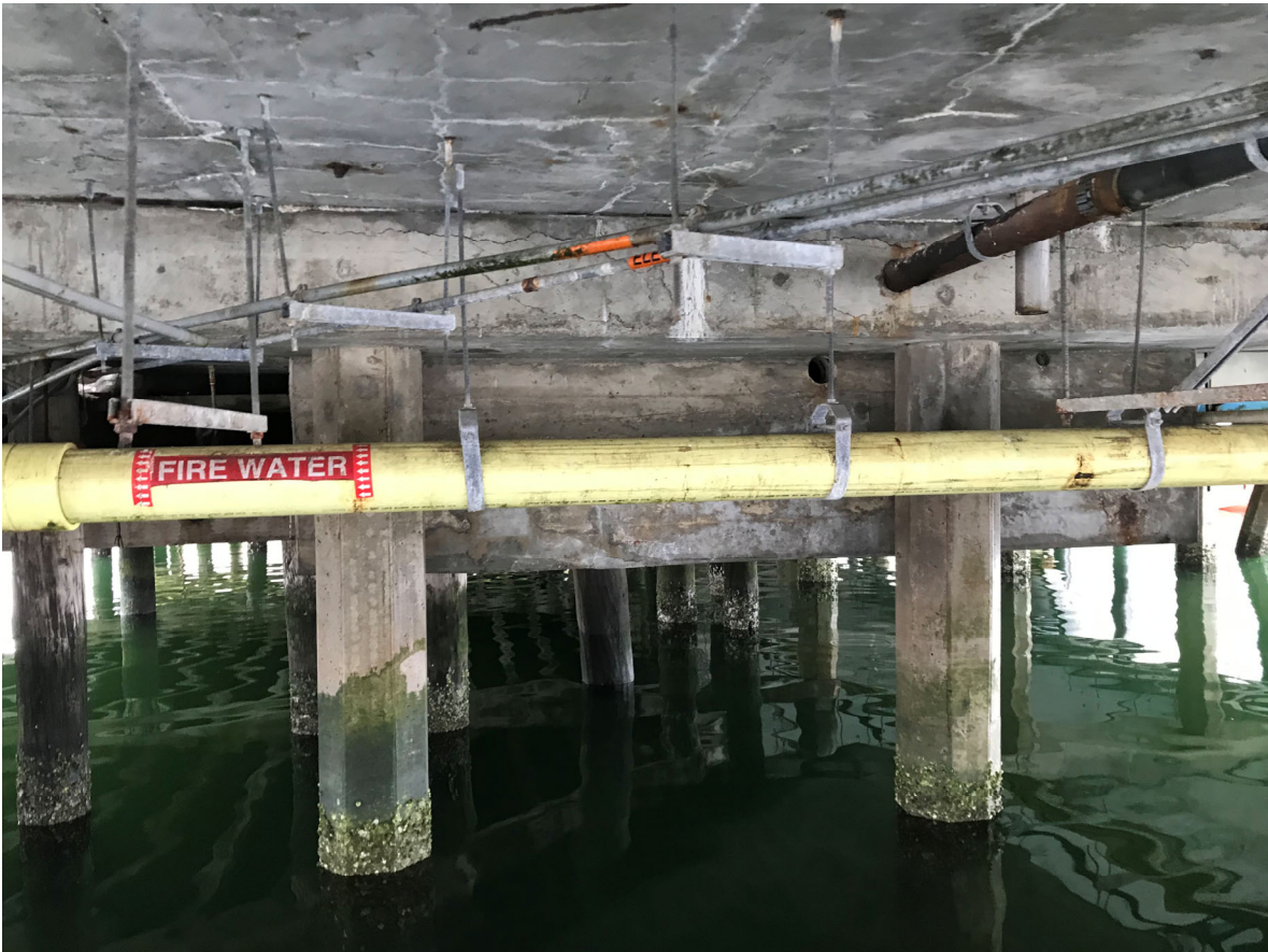
7 – View of overstress cracked beam and utilities under end of pier
