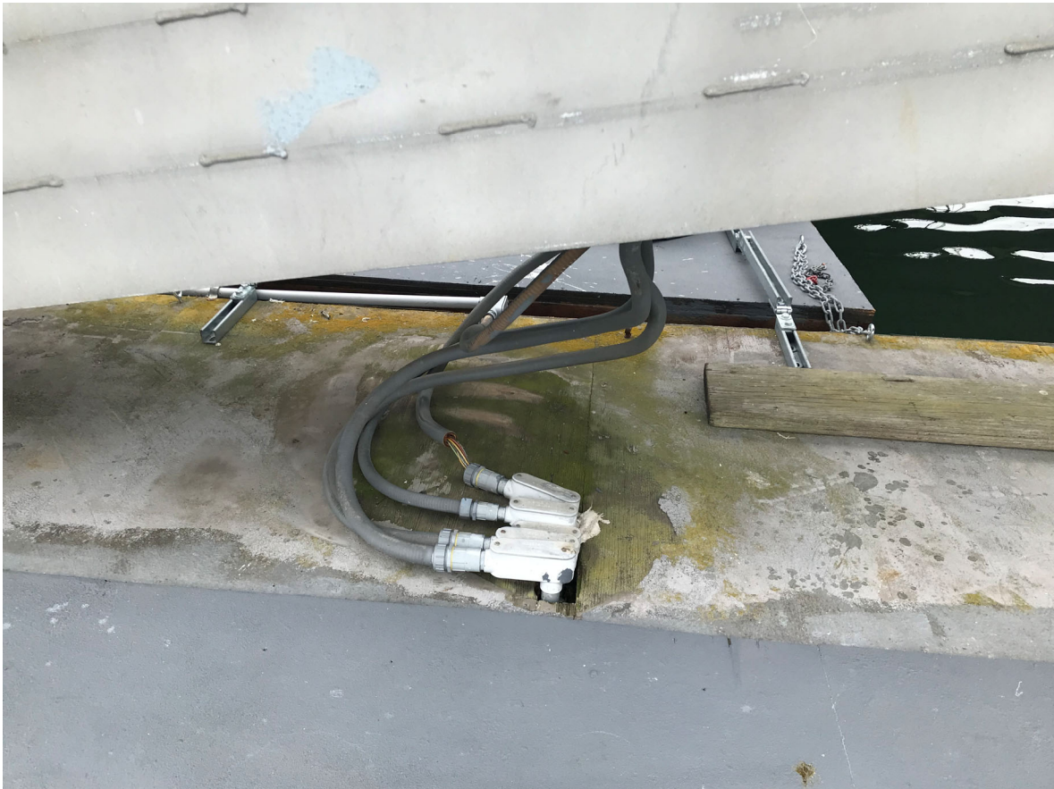
73 – View of electrical to Fuel Dock
