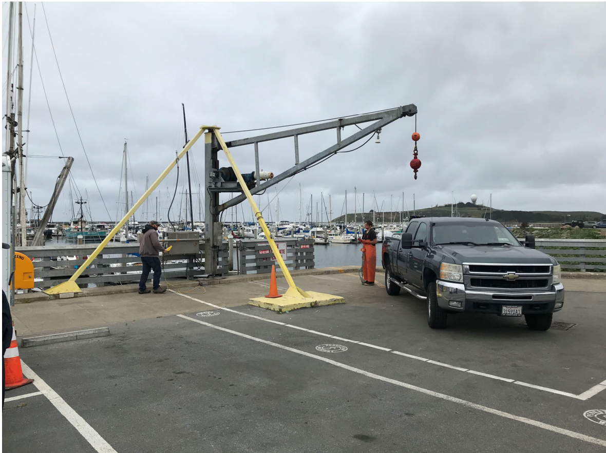
39 – View of public hoist
