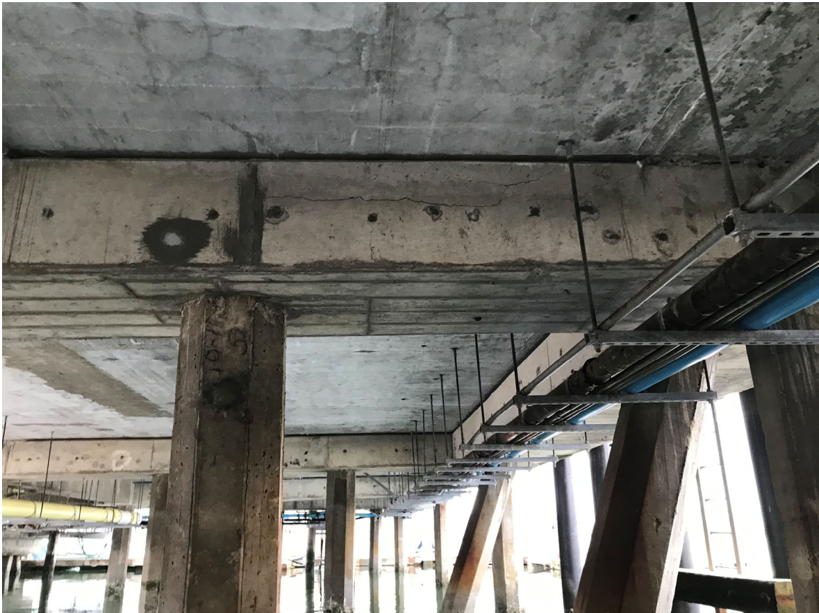
9 – View of overstress cracked beam and utilities under end of pier
