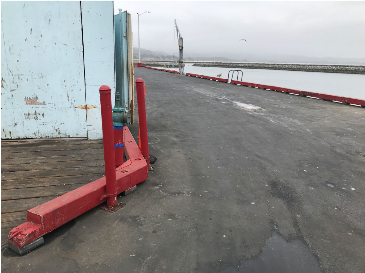
13 – View of high traffic area of pier deck next to Fish Buyer Building
