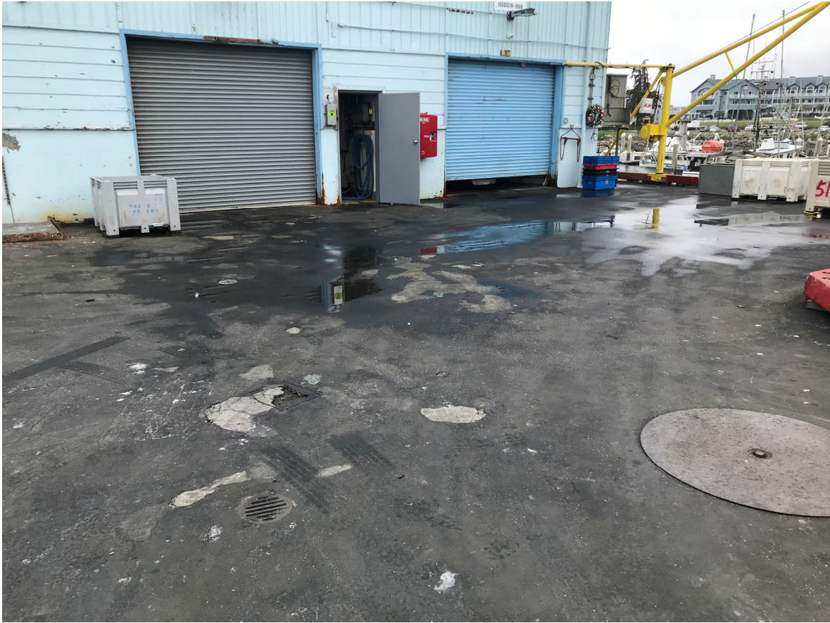
12 – View of high traffic area of pier deck next to Fish Buyer Building
