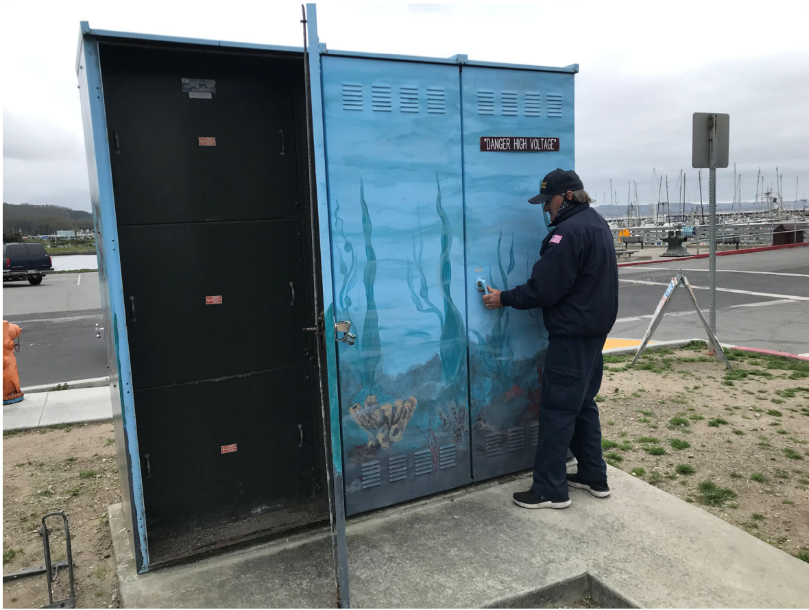
38 – View of main harbor distribution panel from Edison transformer
