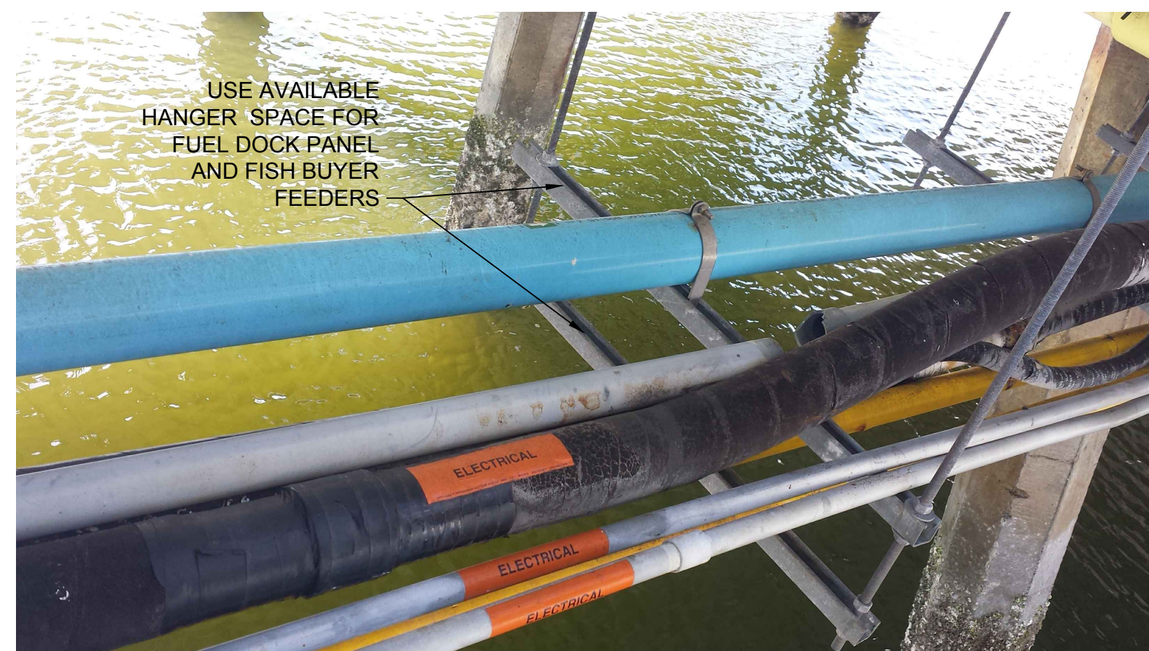
4 EXISTING EAST SIDE PIPE HANGERS EP01 SCALE: NTS
